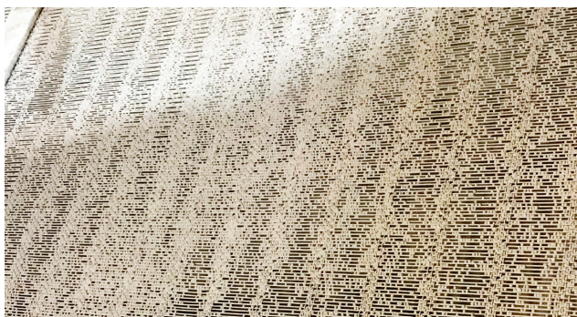
Figure 2. Blinded screen wire mesh.
